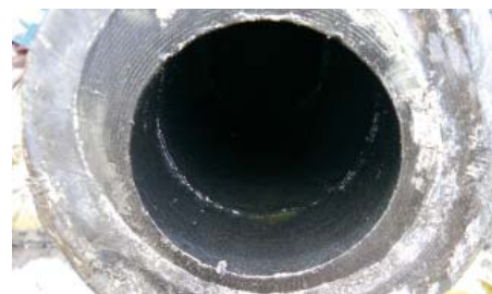
Thermoflow® treated pipeline
